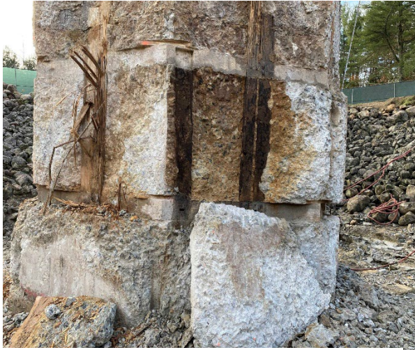
Splintering of wooden timbers
